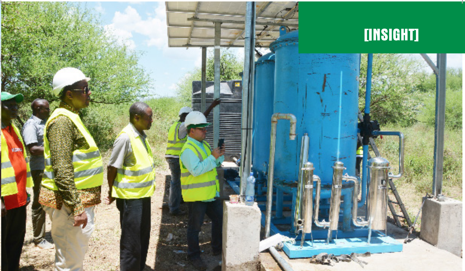
Water for community...Chairman of the GDC Board of Directors Mr. Gershom Otachi Bw'Omanwa (center) and Managing Director & CEO Eng. Johnson P. Ole Nchoe (left), with a contractor at one of the community water filtration points in North Rift
